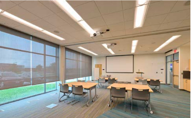
Motorized window shades to control sunlight
