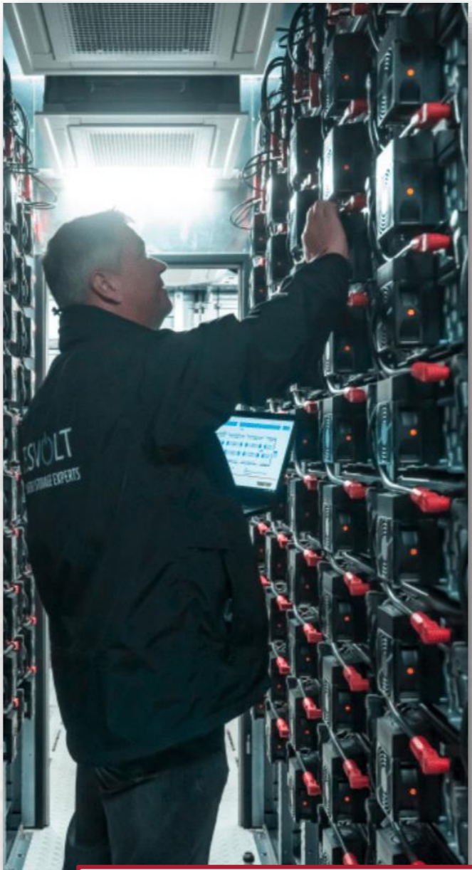
Battery Electric Storage (BES) Emergency power and demand reduction
