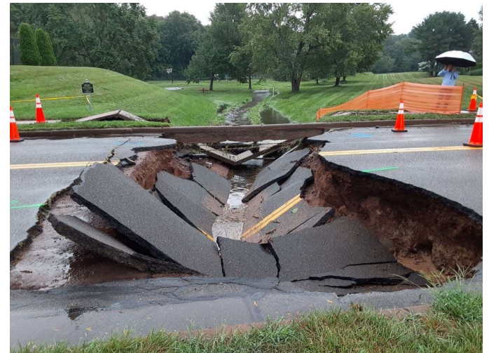
A collapsed portion of Ambassador Drive following Tropical Storm Henri. Source: Patch.com
