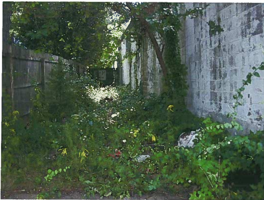
An area of debris is located along the eastern portion of the building
