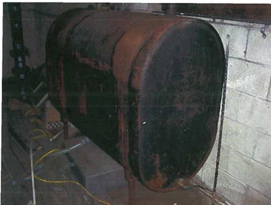
330-gallon fuel oil AST located between the boiler room and storage space
