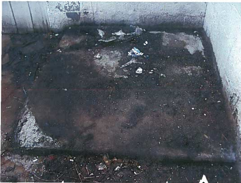
A stained concrete pad located to the north of the heating oil UST
