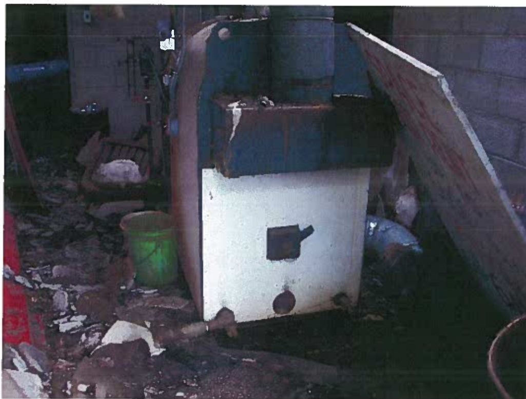
Fuel oil-burning furnace located in the boiler room
