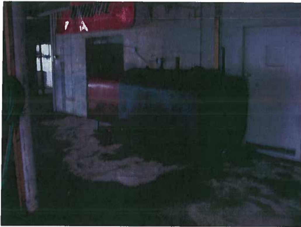
Three used oil ASTs located in the central portion of the former service area
